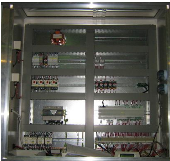
Fig. 13: View of the electrical panel.
